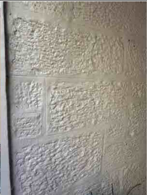
123 Barnard Street Plastic Paint on stone
